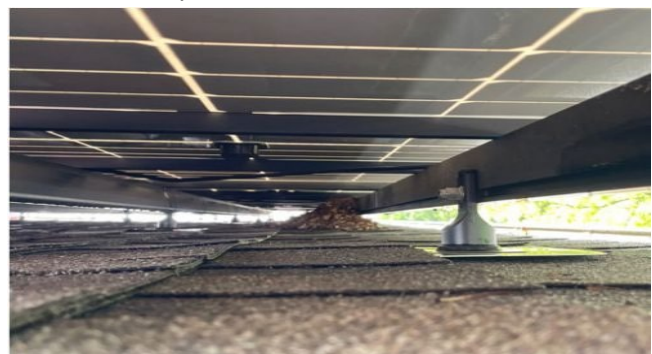
Debris buildup underneath the panels
