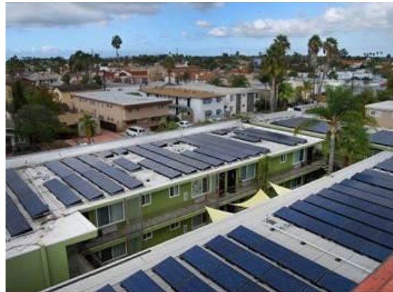
A solar photovoltaic (PV) system atop the 34-unit multifamily affordable housing Townspeople Apartments in San Diego provides 88% of its production to tenants. Photo courtesy Center for Sustainable Energy 858-244-1177
